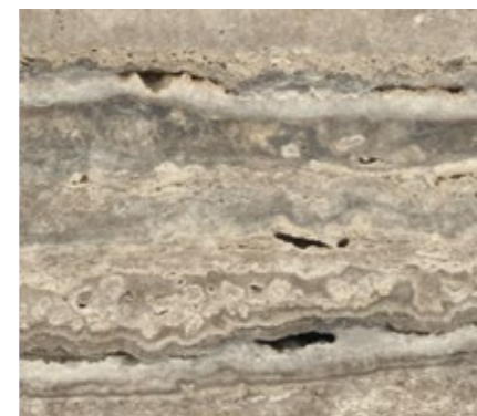
stuccatura a mastice o resinatura (dettaglio) plastered with mastic or resin-treated (detail)
